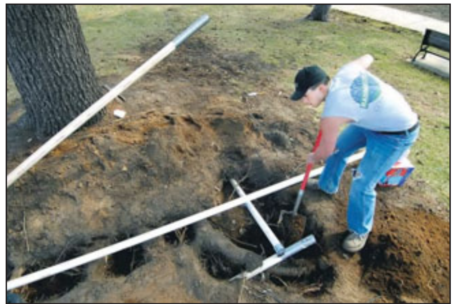
Staff photo by Dan Reiland RainMaster Lawn Systems employee John Stricklin dug around tree roots in Wilson Park on Wednesday to install a new sprinkler system. The Eau Claire Parks, Recreation and Forestry Department is paying $9,000 for the new equipment, and officials hope weather-sensing technology controlling the sprinklers will save on water and labor.
